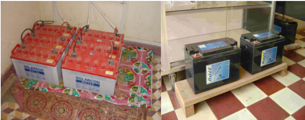
Picture 37: Battery storeroom
