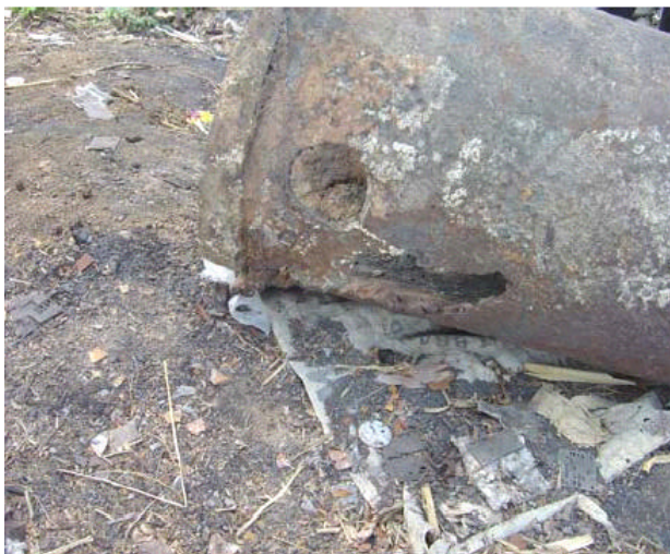
Picture 31: The corroded furnace tube
