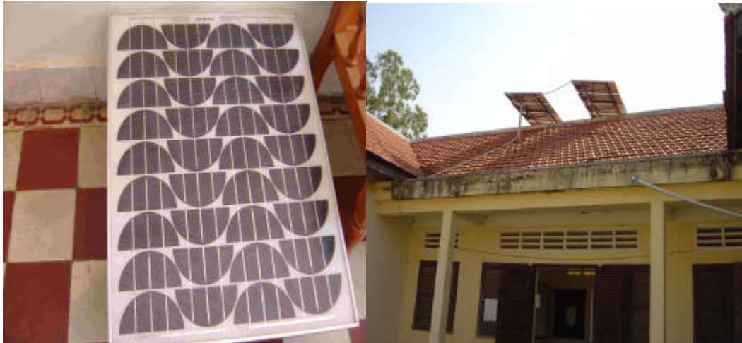
Picture 35: RAPS installed at a public school in Svay Rieng province
