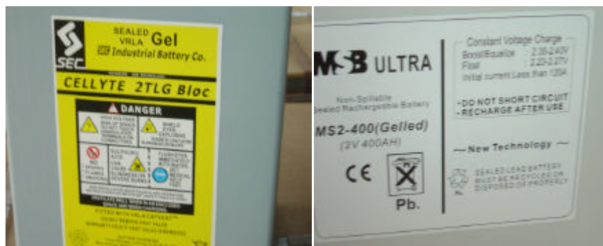
Picture 38: Valve Regulated Gelled Batteries
