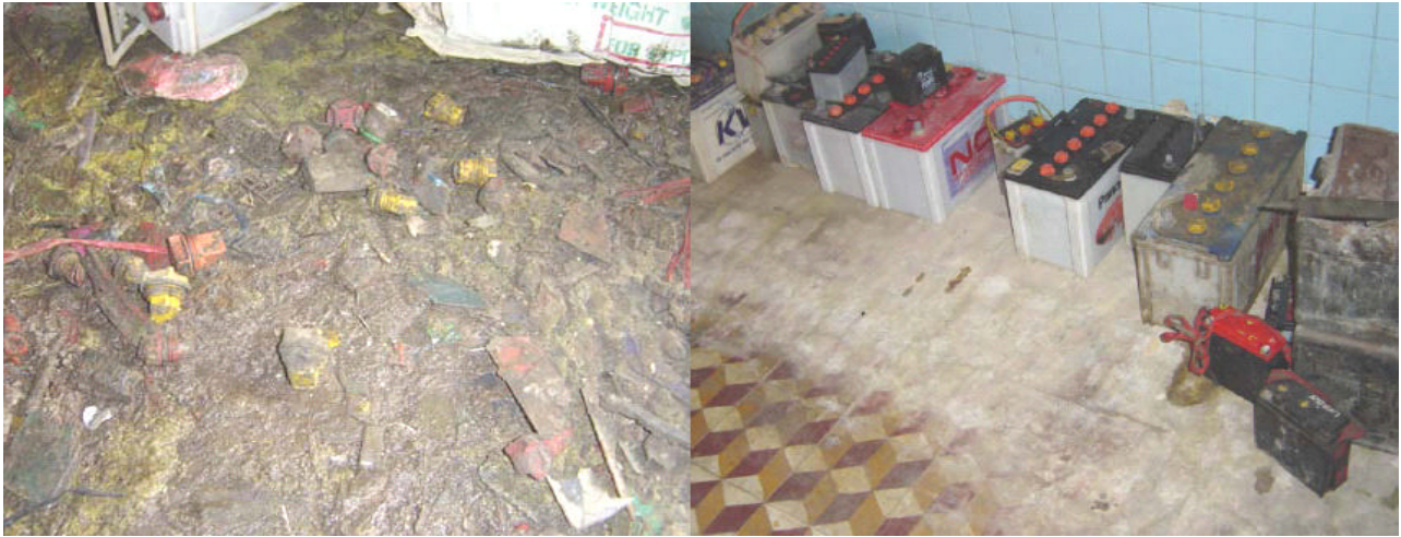
Picture 16: Acid spillage on soil and paved floor storerooms
