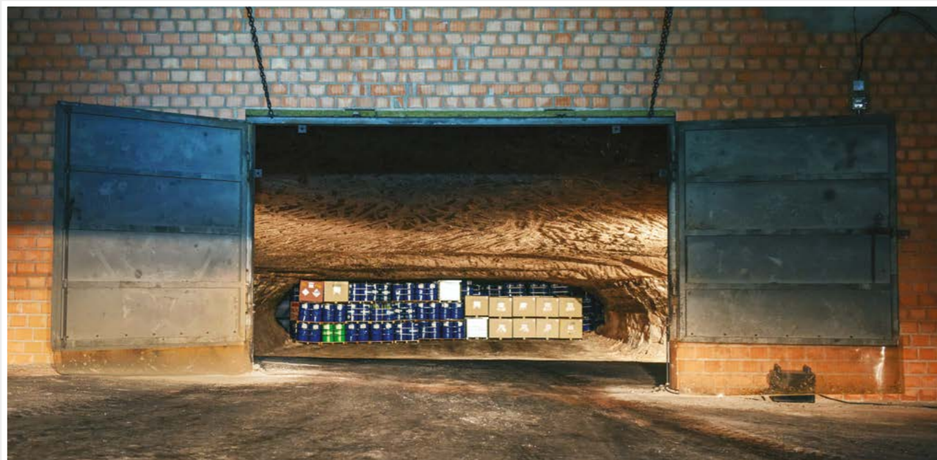
Disposal chamber for mercury-contaminated wastes in the underground facility © K+S Entsorgung GmbH
