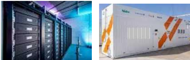
Figure 2: Battery Energy Storage System (BESS)
